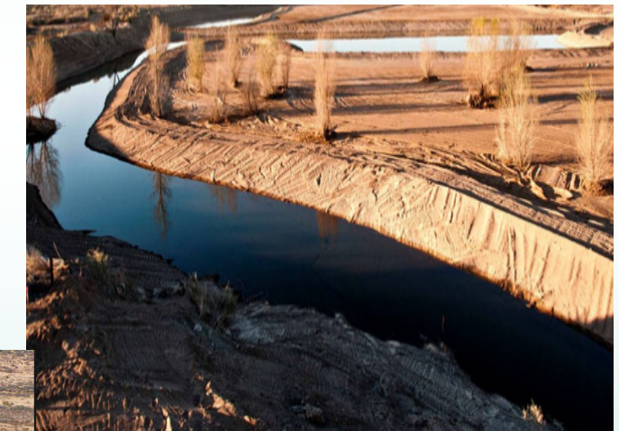
Left: Photo of construction in progress at Hunters Hole Conservation Area in 2012.
